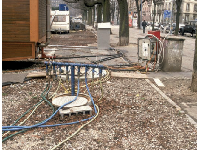
Figure 18 : Câblages "spaghetti". Source : Carlos Lopez
