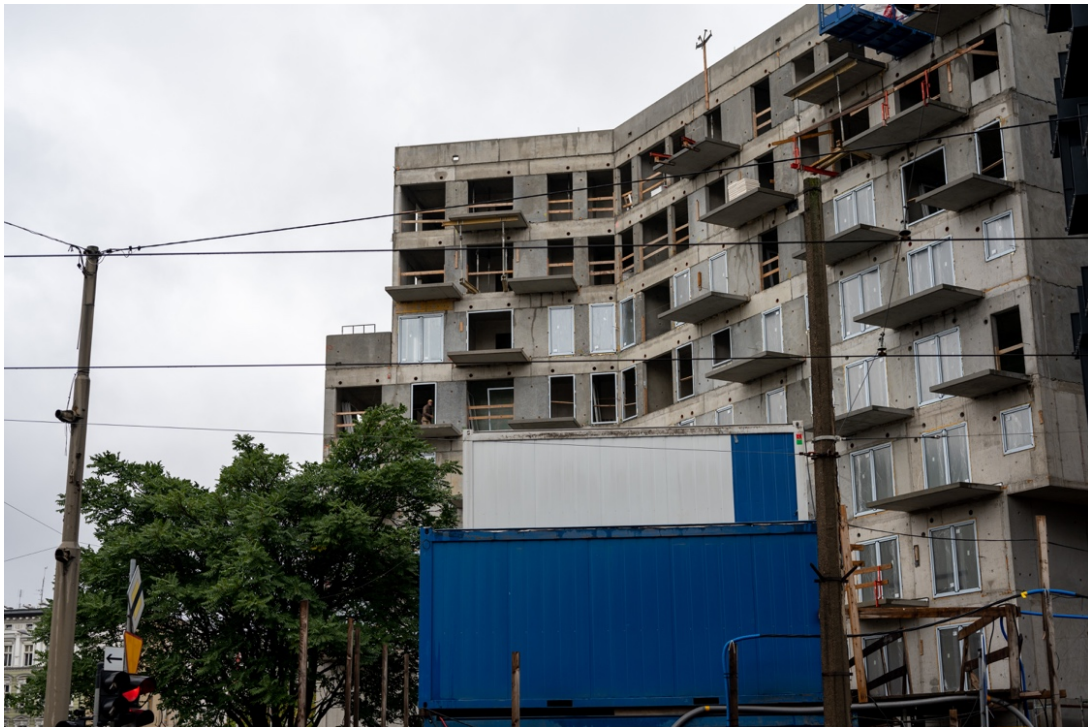
Figure 1 – A new allotment in construction in the district of Przedmieście Olawskie. Photograph: Benjamin Péry, 2021.
